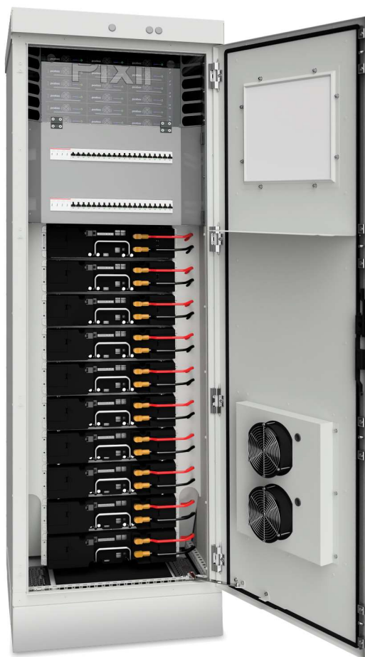
PowerShaper 30kw / 65kWh
